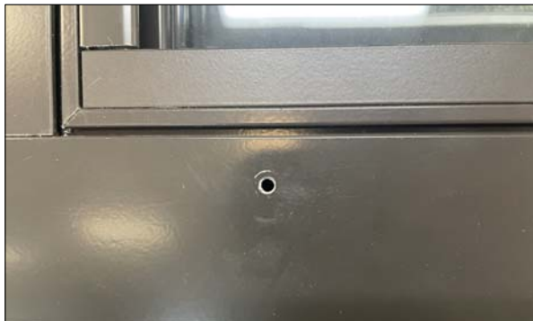
EXPOSED \frac{3}{16} " HOLE WITH SCREEN CLIP REMOVED
